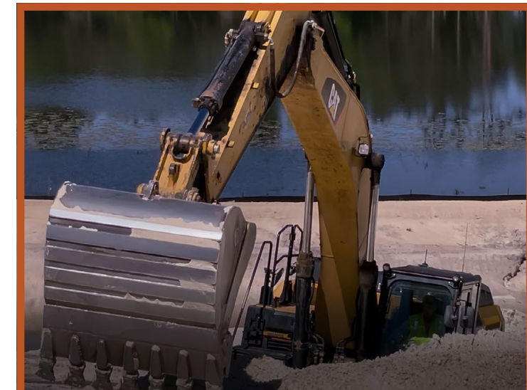
Excavators provide impressive muscle power and are being used to construct eight stormwater ponds, including the pond site south of Rolling Pines Road and Pine Ridge Drive.
