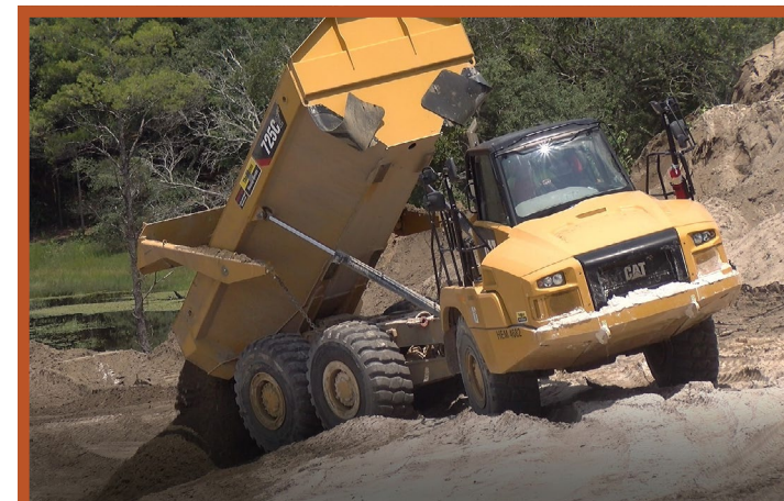
Off-road dump trucks are fitted with hydraulic mechanisms which unload materials with ease during pond site construction, reducing operation costs.
