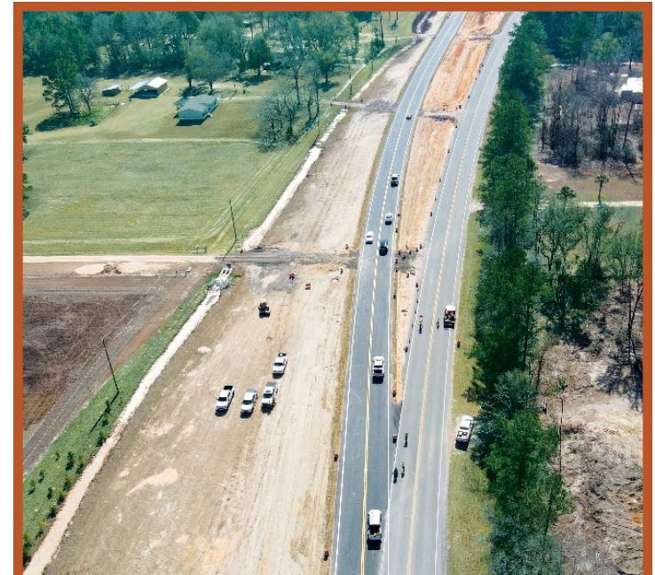
North and southbound traffic between Sunny Hills Boulevard and Rogers Road shifted to the newly constructed northbound lanes in February.
