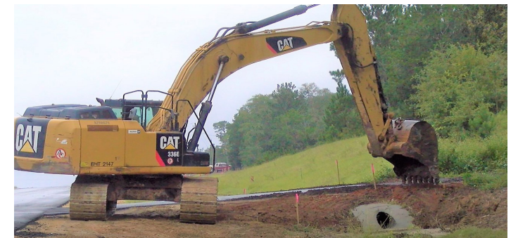
(TOP and MIDDLE) Crews add drainage improvements near Pompey Avenue in the city of Vernon.
